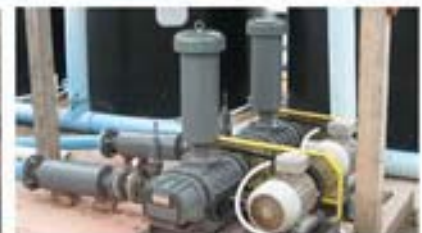
Waste water treatment
