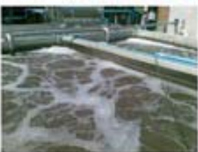
Waste water treatment
